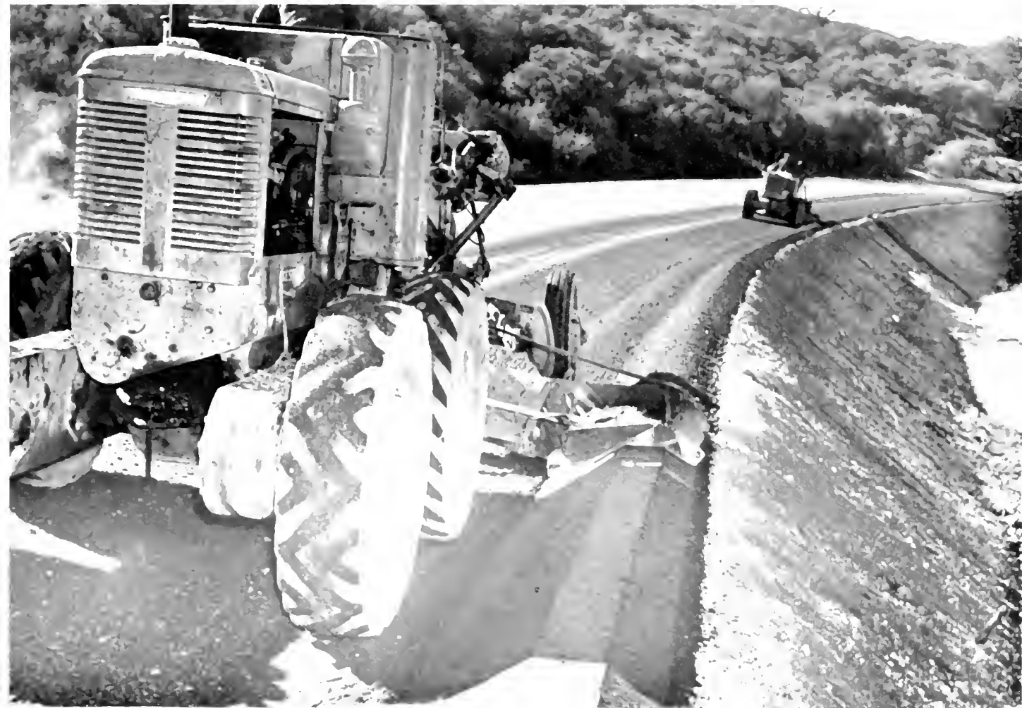
Picture of dozer spreader with spreader-box blade attachment constructing plant-mixed berm and gutter
